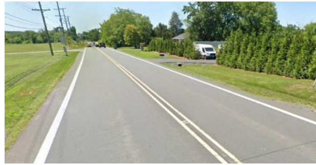
Center Line Pavement Markings (Example Location: Leesburg, VA)
